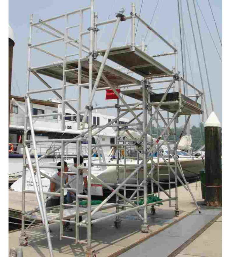
Special tower for yacht maintenance
